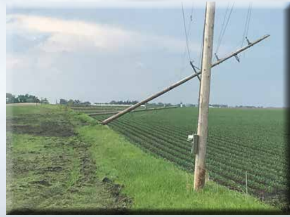
High winds took down transmission lines south of Hanska on Memorial Day.
